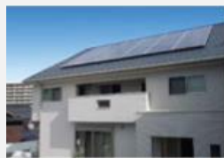
Residential solar power generation system
