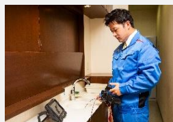
Endoscopic inspection of the inside of the water supply and drainage pipes
