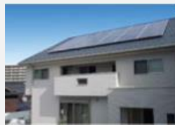
Residential Solar Power Generation System
